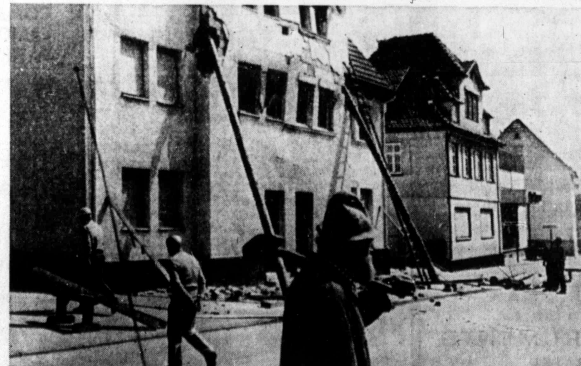
QUAKE DAMAGE—Outside walls of a home in Albstadt, West Germany, are propped up by heavy poles after an earthquake, reading over 7 on the Richter Scale, rumbled through the area early Sunday. The quake, which rocked southwestern Germany, eastern France, northern Switzerland and western Austria, caused damage estimated in the millions of dollars. (AP Laserphoto)
