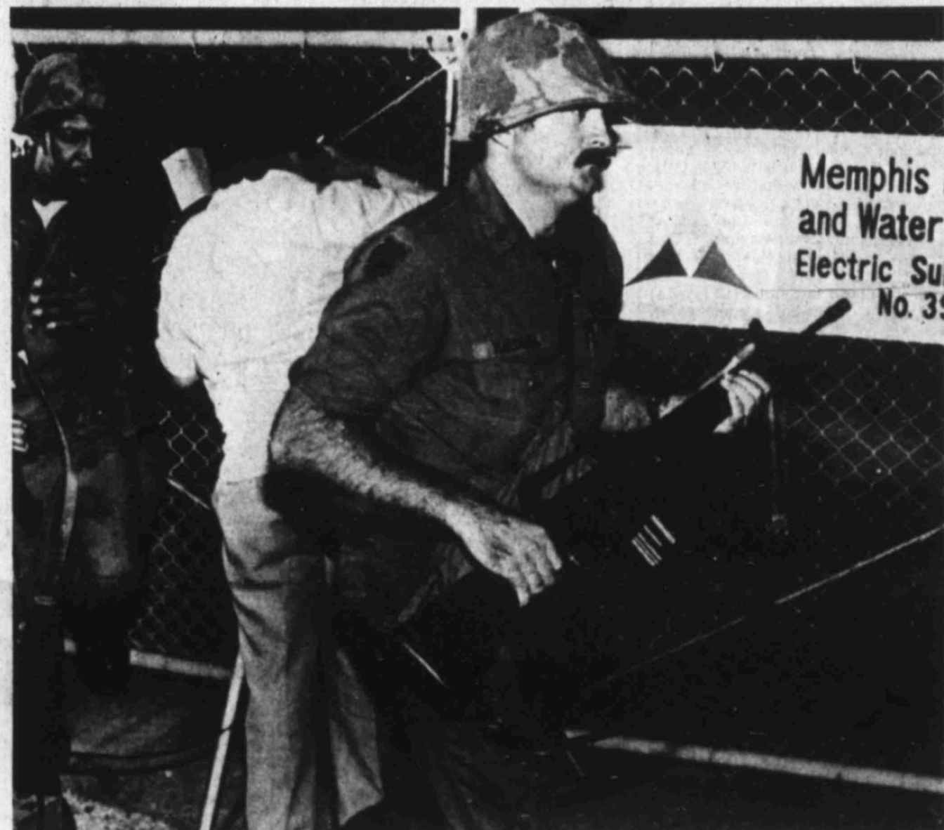
TENNESSEE NATIONAL GUARDSMEN take up positions at the Cordova power substation in Memphis early today after a blackout plunged the city
