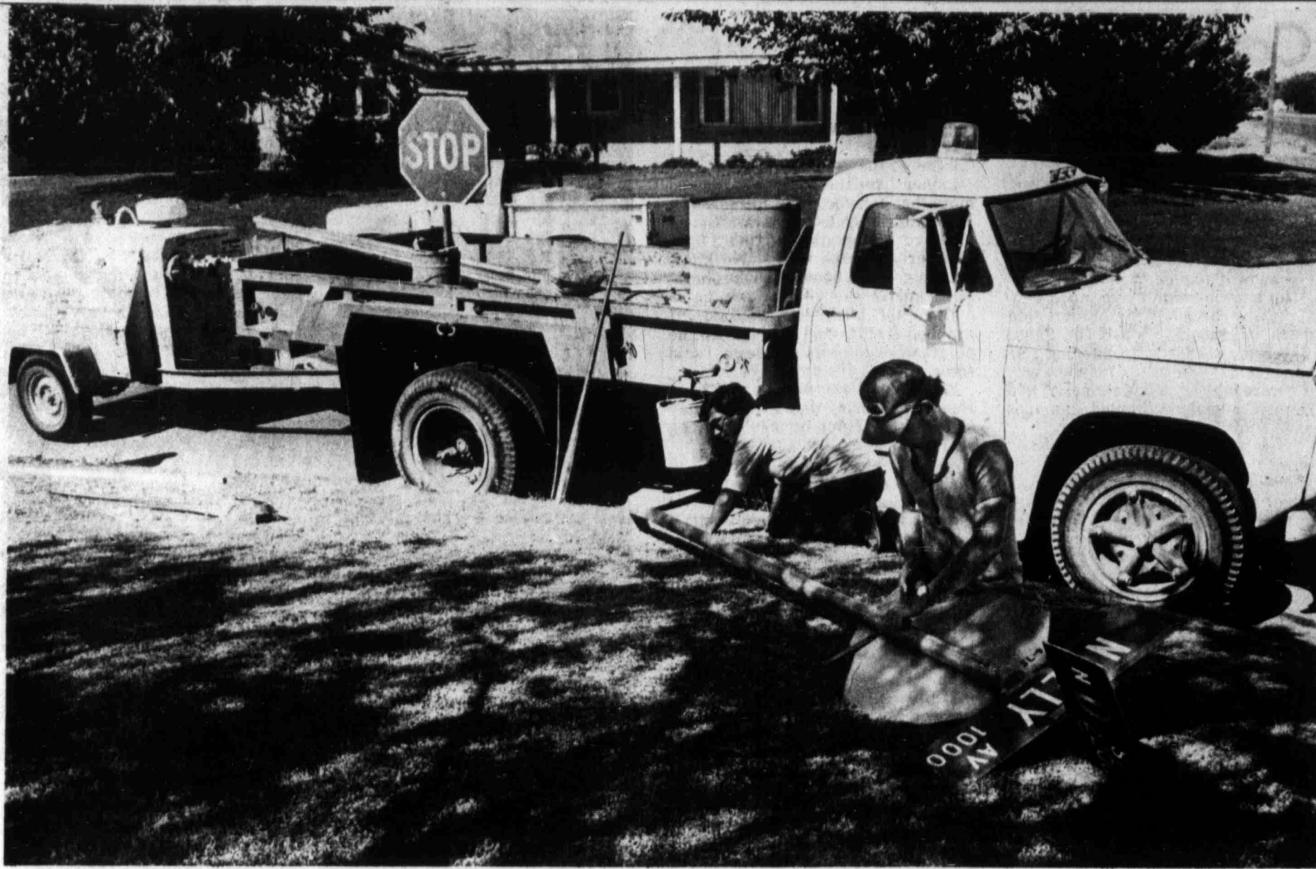
CITY CREWS have been busy lately repairing some 22 stop signs that were bent recently. Rudy Carrasco, left, and Loyd Miller work on one of the signs at the intersection of Neely and D streets. (Staff Photo)
