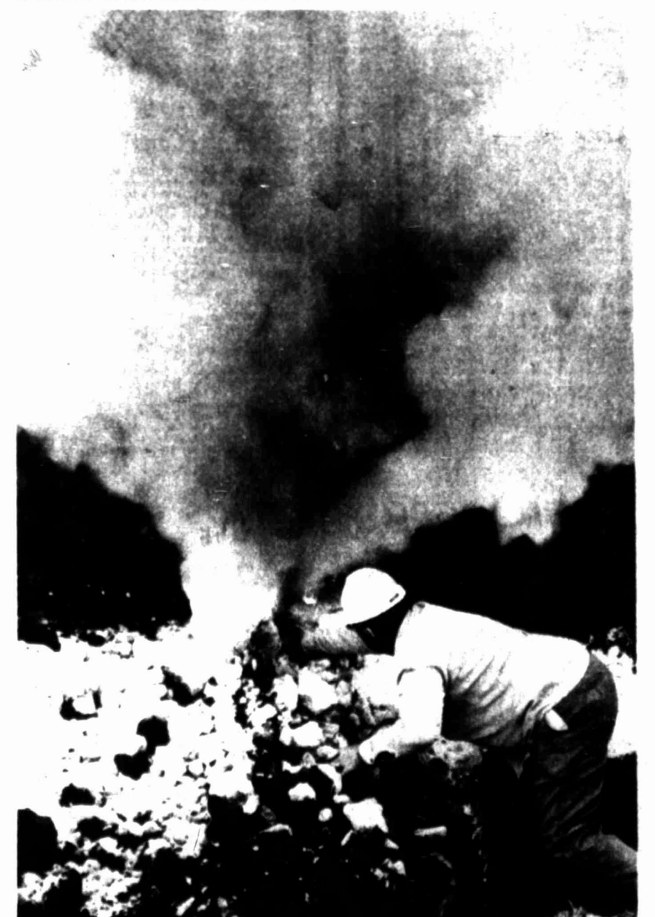
ESCAPING GAS billows out of a deep hole where a dead horse was to be buried on the Midland Polo Club grounds this morning. A front-end loader digging the hole struck a liquified petroleum gas line, causing the leak. Clarence Gallagher, employed by Mobile Pipeline Co., inspects damage to the eight-inch line. Related story on Page 3A. (Staff Photo By Mike Kardos)
