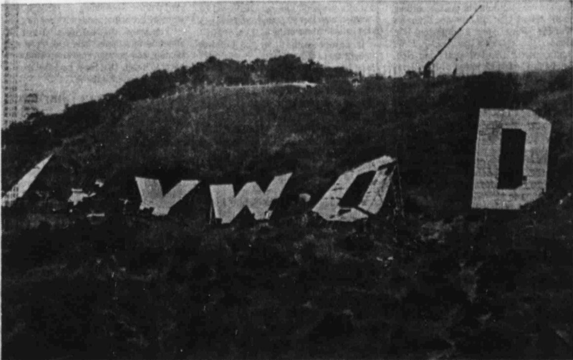
FAMED LANDMARK COMES DOWN — Workmen prepare to lower the last letter in the famed "HOLLYWOOD" sign that has stood in the hills overlooking Hollywood and Los Angeles for several decades. The old sign, made from telephone poles
