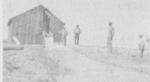
BRINGING IN A WELL. Pictured here are (left to right) Frank Johnson, Mr. Teidy of Bovina, E.H. Buhrman and sons Russell and Cecil. This was the first irrigation well of its type in this part of Texas. Land agents used to hold water carnivals to promote land sales in Bailey County.
