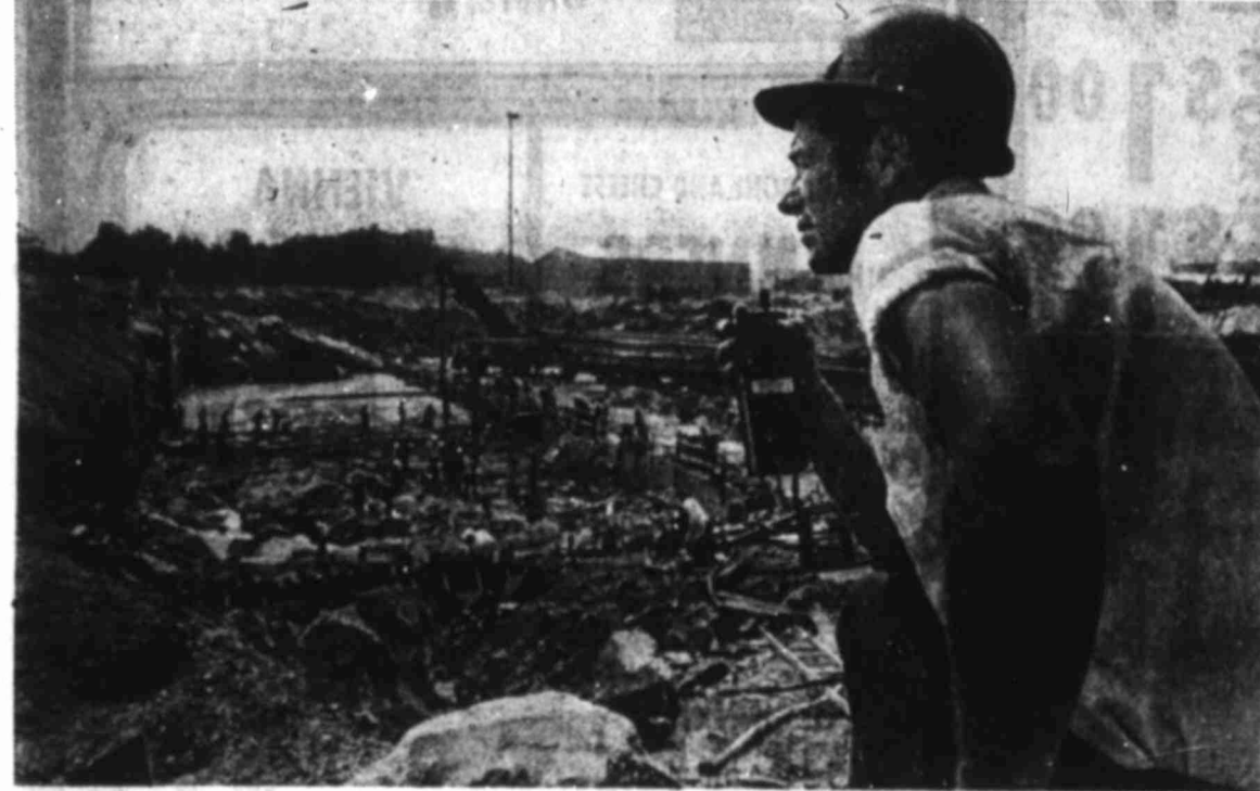
NUCLEAR POWER CONSTRUCTION — As the final day of construction ends Friday at the Seabrook nuclear power plant, a superintendent of construction, Jeff DiBiasco, watches the last batch of concrete being poured into the base pad of the cooling towers for the nuclear reactors. With the construction permit pulled by the Nuclear Regulatory Commission, work on the nation's largest atomic power generator came to an end at 6 p.m. Friday. (AP Laserphoto)
