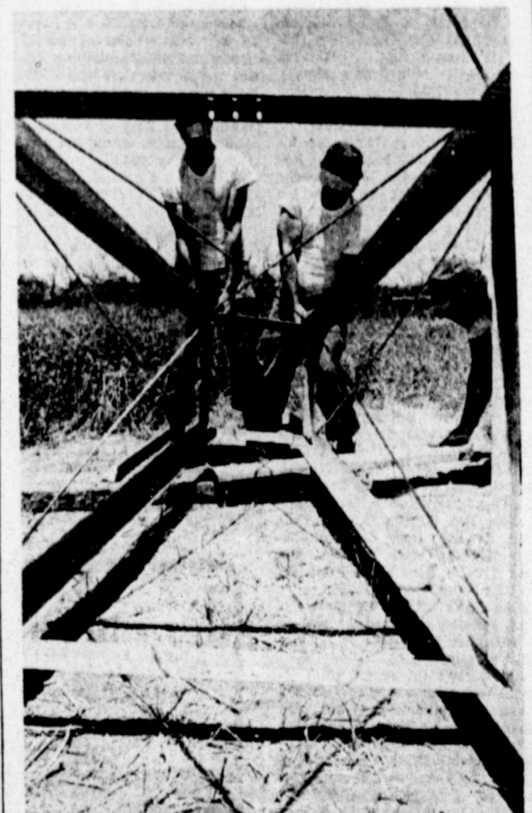
Cpts. Rayce Swayne and Tammy Boyd struggle with the top of a windmill being built by the Army Reserve for a girl's foster home.
