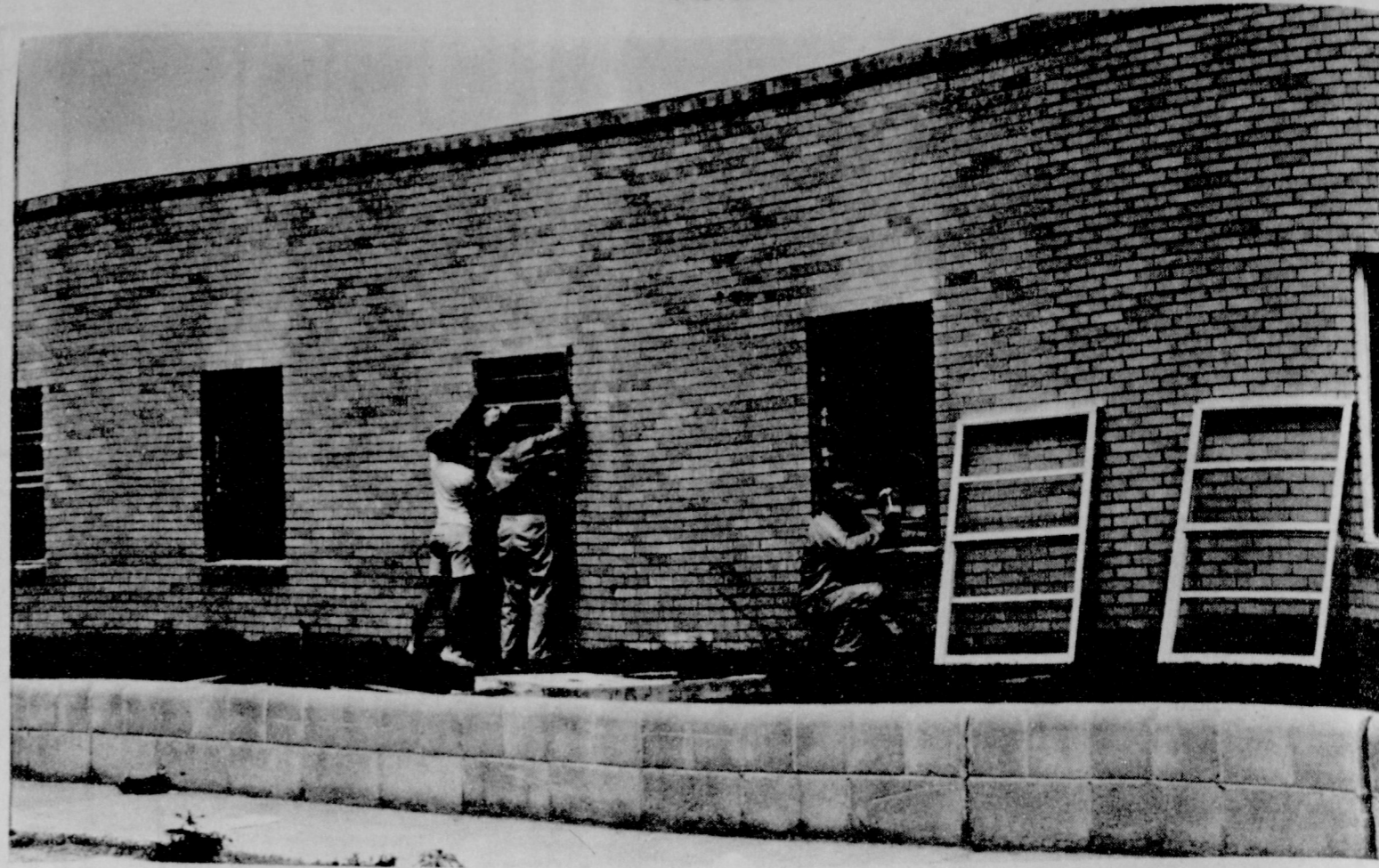
NEW WINDOWS— West Plains Hospital and Clinic is installing metal-frame windows in the place of wooden frames, and here workers are shown at work on the job, a "quickie operation" since patients had to be moved to the other side of the hospital as the windows were being replaced. Note bed still in room in foreground. (Journal Photo)
