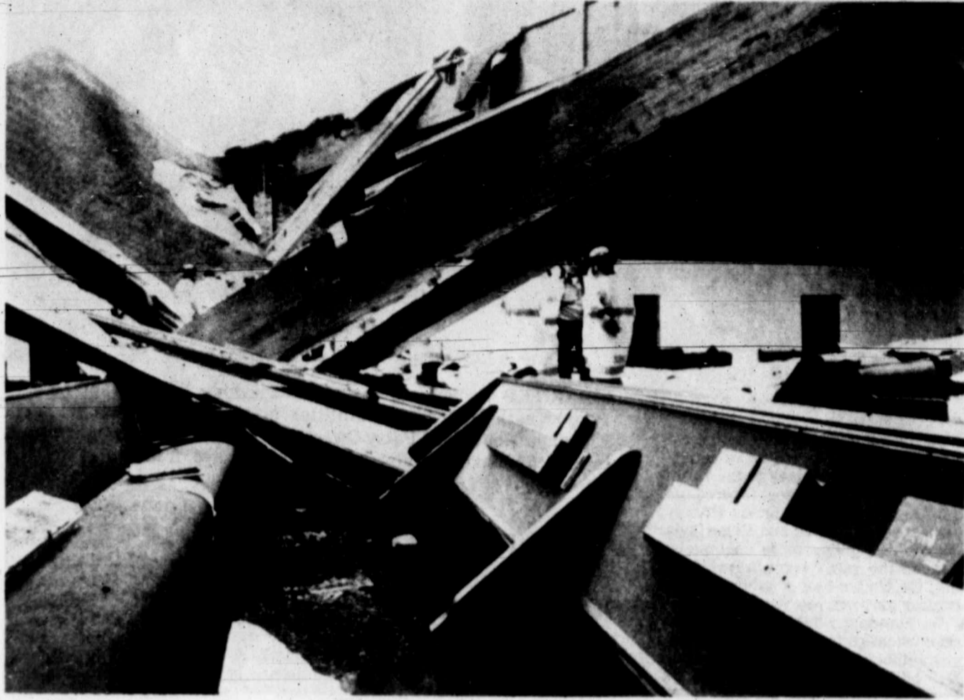
Fire and rescue workers sift through debris Sunday after roof of Walnut Village Church of Christ collapsed during services, killing one. Police
