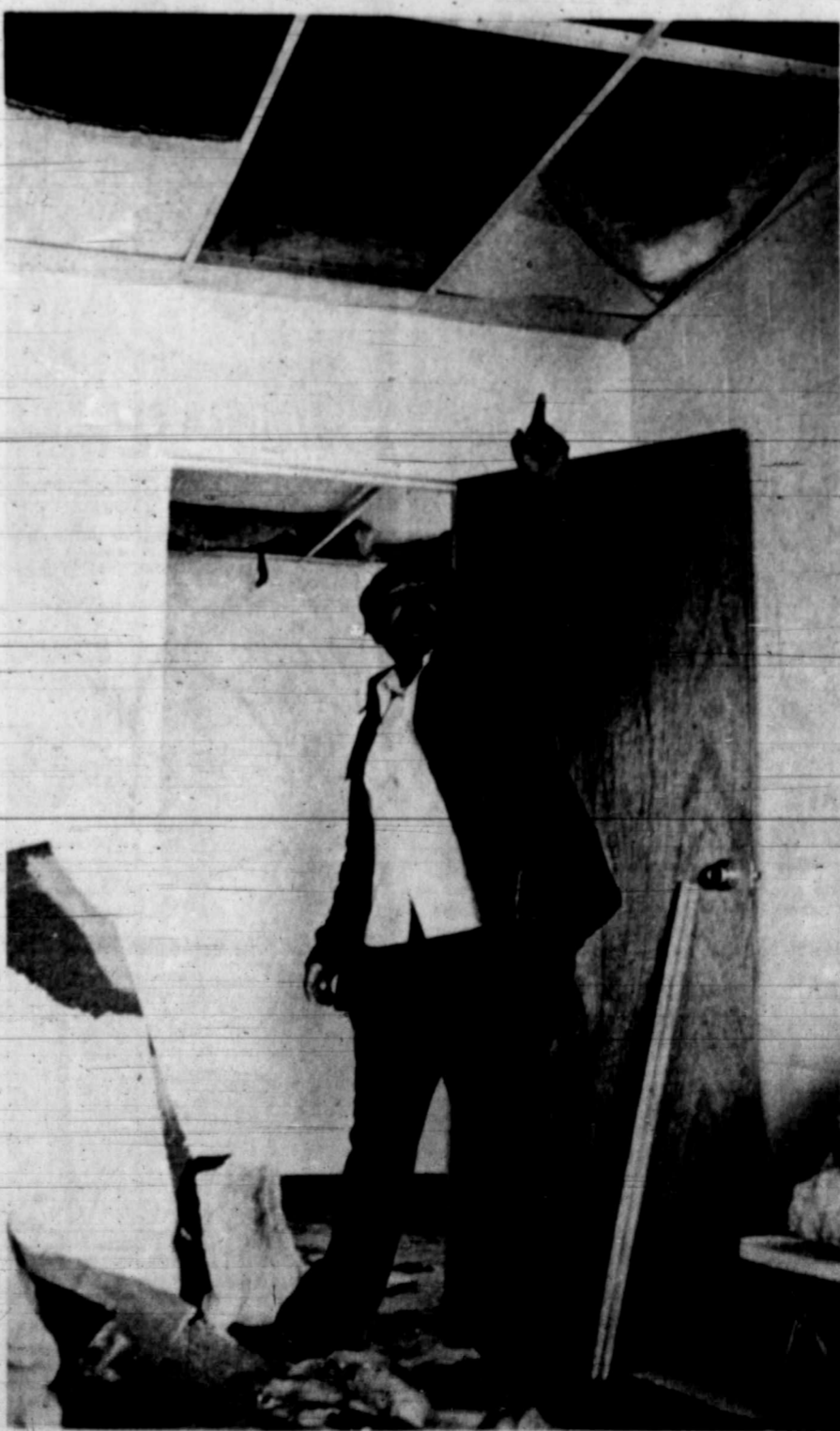
Emilio Sanchez points skyward to the rain damage done to the ceiling at the Midland Latin Free Methodist Church Tuesday morning. (Staff Photo)
