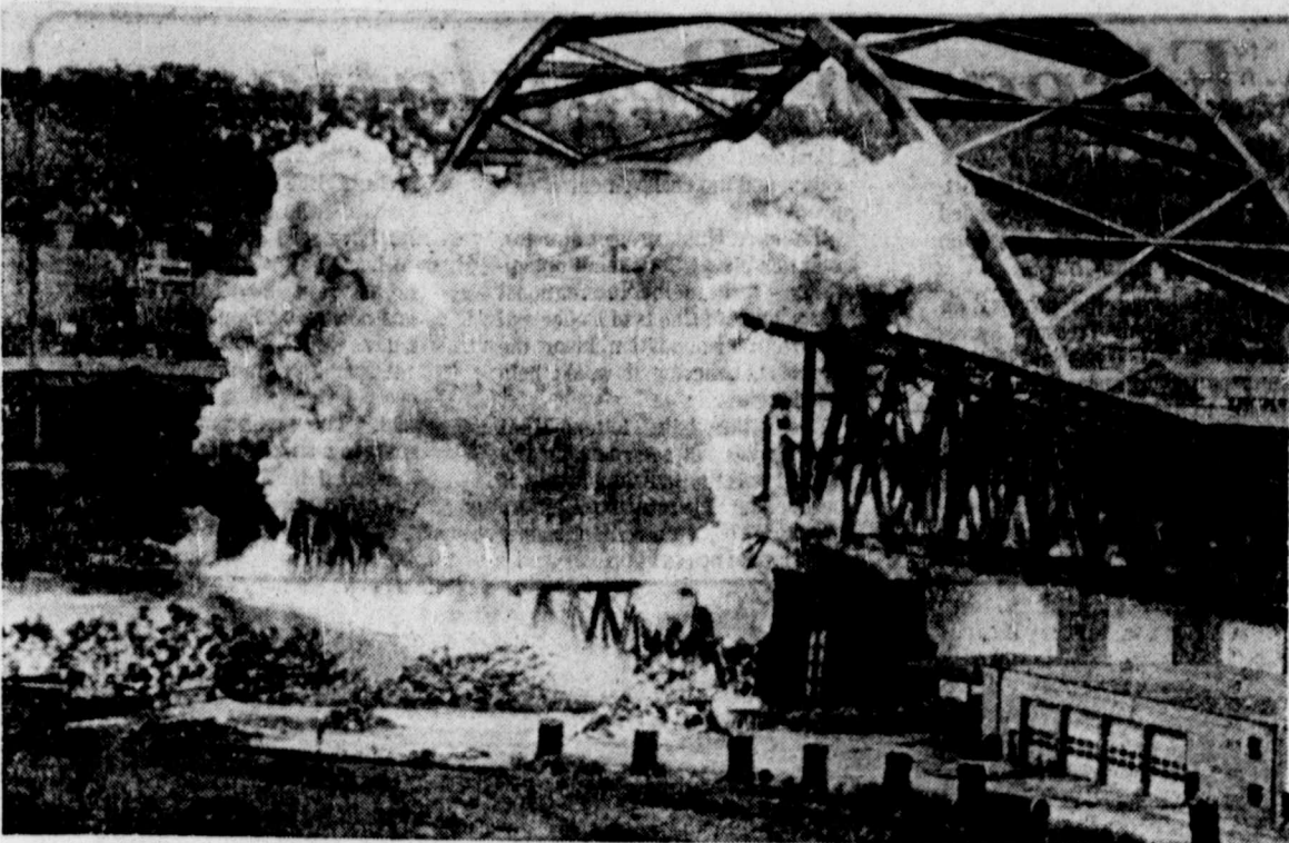
IN THE RIVER — The center span of the Brady St. Bridge in Pittsburgh splashed into the Monongahela River Monday night. The 67-year-old bridge was destroyed by demolition experts using explosives. The south span also fell, but the north span remained. (AP Laserphoto)
