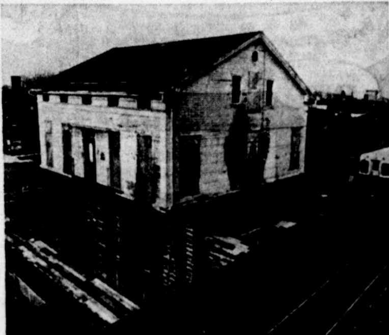
JACKS CREATE HIGH-RISE—Henry B. Clarke House, oldest house in Chicago, is perched 25 feet above ground before its next move—over the elevated tracks. House is making a $410,000 move from its former location to a historic district. Workmen hope to move the 150-ton house over the tracks early Sunday morning while there is little activity. (AP Laserphoto)
