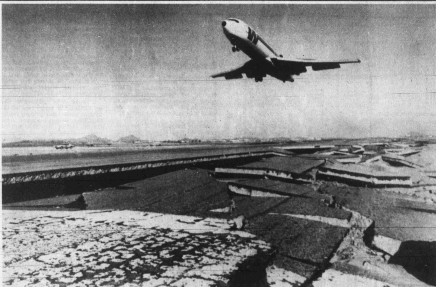
IT'S BUSINESS AS USUAL at Phoenix Sky Harbor International Airport Wednesday despite condition of east end of main runway. Repairs are estimated at $4 million. (AP Laserphoto)
