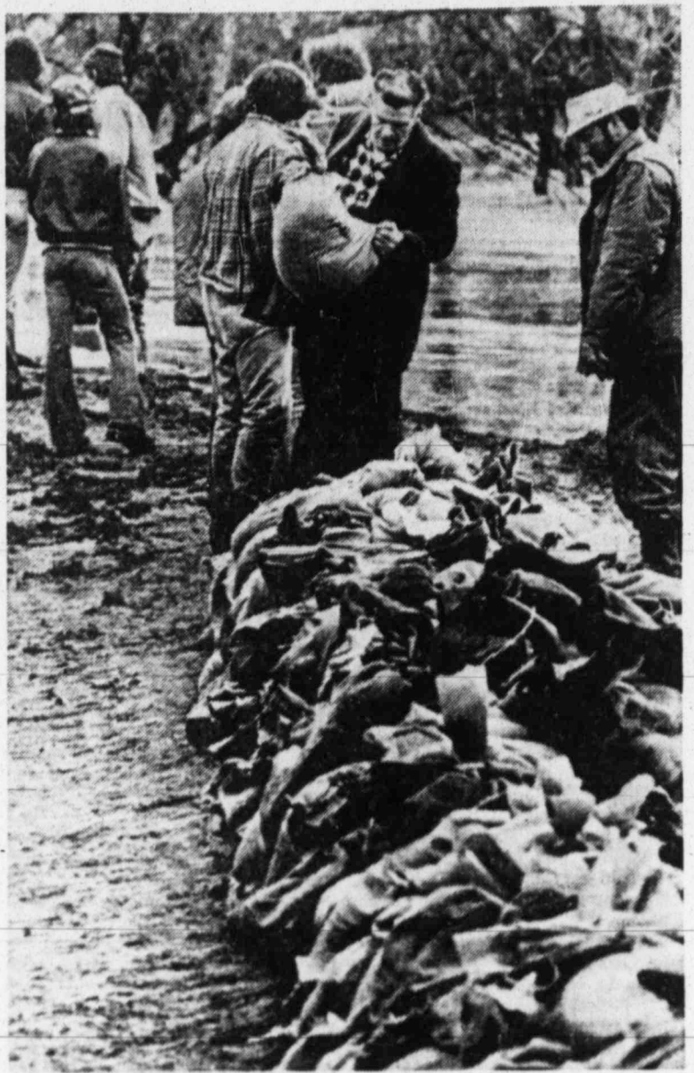
WORKING ON DIKES — Volunteers at East Grand Forks, Minn., reinforce dikes Sunday in preparation for a predicted 47-foot flood crest on the river Wednesday. The National Guard was called out to help the residents of the town. Warm weather has triggered flash floods in the upper Midwest. (AP Laserphoto)
