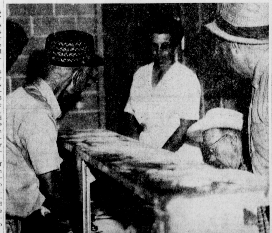
Here a crew of workmen are installing equipment in the brand-new senior-junior cafeteria. (Journal Photo)
