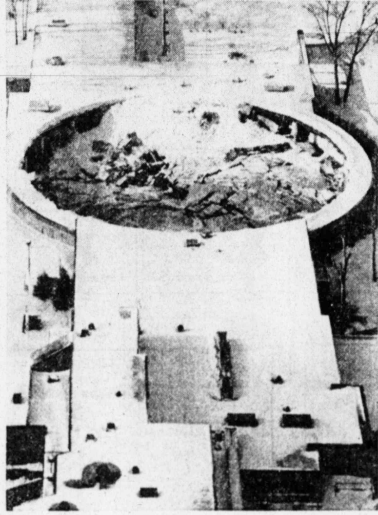
ROOF CAVED IN — The collapsed domed roof of the 3,000-seat auditorium on the campus of C.W. Post College in Brookville, N.Y., presents a bomb crater vision in this overhead view. Police said the roof, made of steel and fiberglass and measuring 300 feet in diameter, apparently gave way under an accumulation of ice and snow. The building was empty and no one was injured. (AP Laserphoto)
