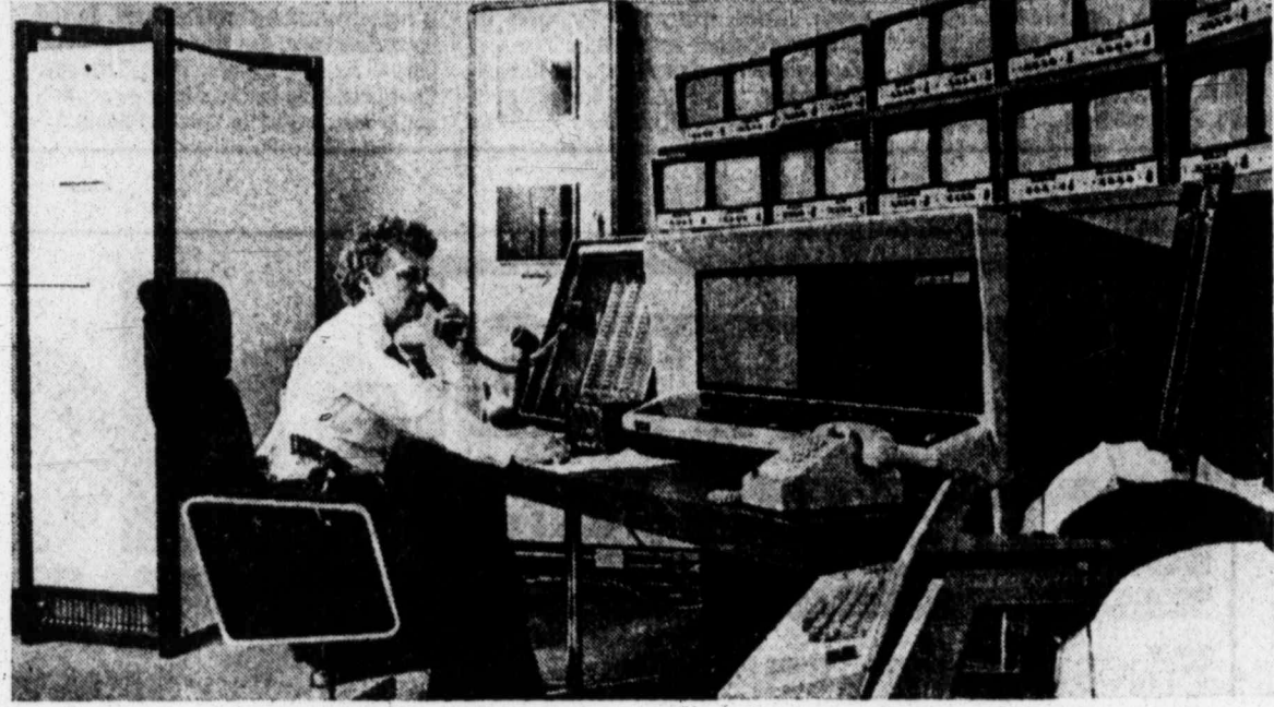
TYPICAL OF LOCAL INSTALLATIONS — Robertshaw operating automation for buildings, as shown here in part, is one of the available services and products from A & C Alarm, a total concept Lubbock firm.
