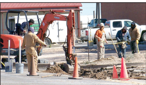
Workers prepare the west side parking lot at Muleshoe State Bank for asphalt.
