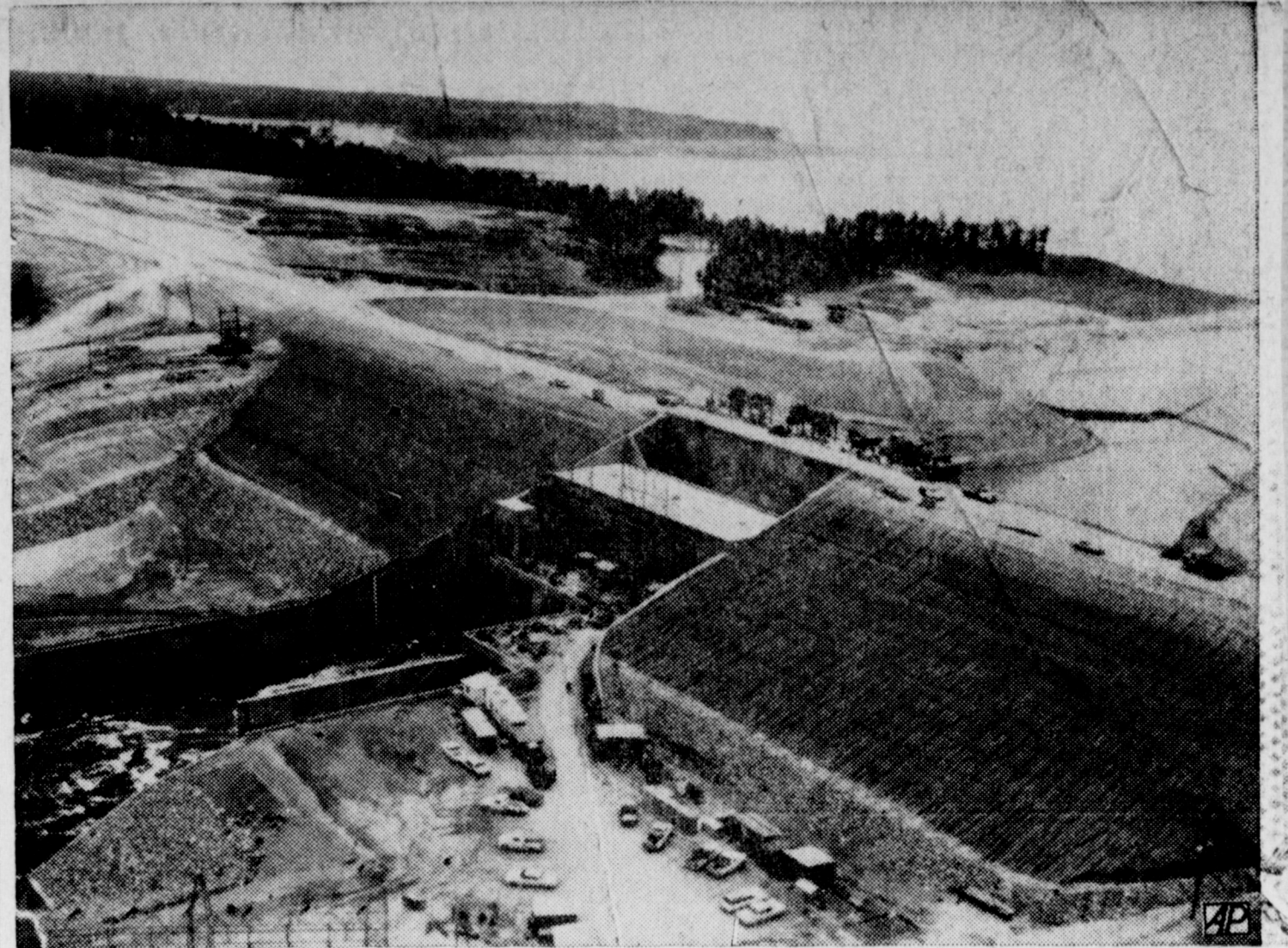
SAM RAYBURN DAM - This is the power plant and outlet structure at Sam Rayburn Dam and Reservoir on the Angelina River 10 miles northwest of Jasper, Tex., which will be formally dedicated May 8. The reservoir, now collecting water, will cover 114,500
