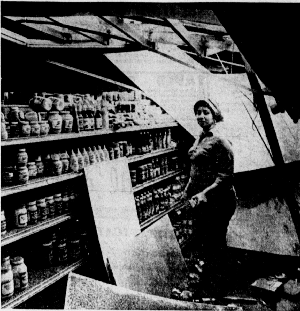
LOSES GROCERY STORE — Angelina Padilla, 30, is pictured standing in the ruins of her new grocery store which was to open this week. The roof collapsed into the center of the store and mounds of sand and debris blocked the aisles after the windstorm this week which swept through much of California. (AP Laserphoto)
