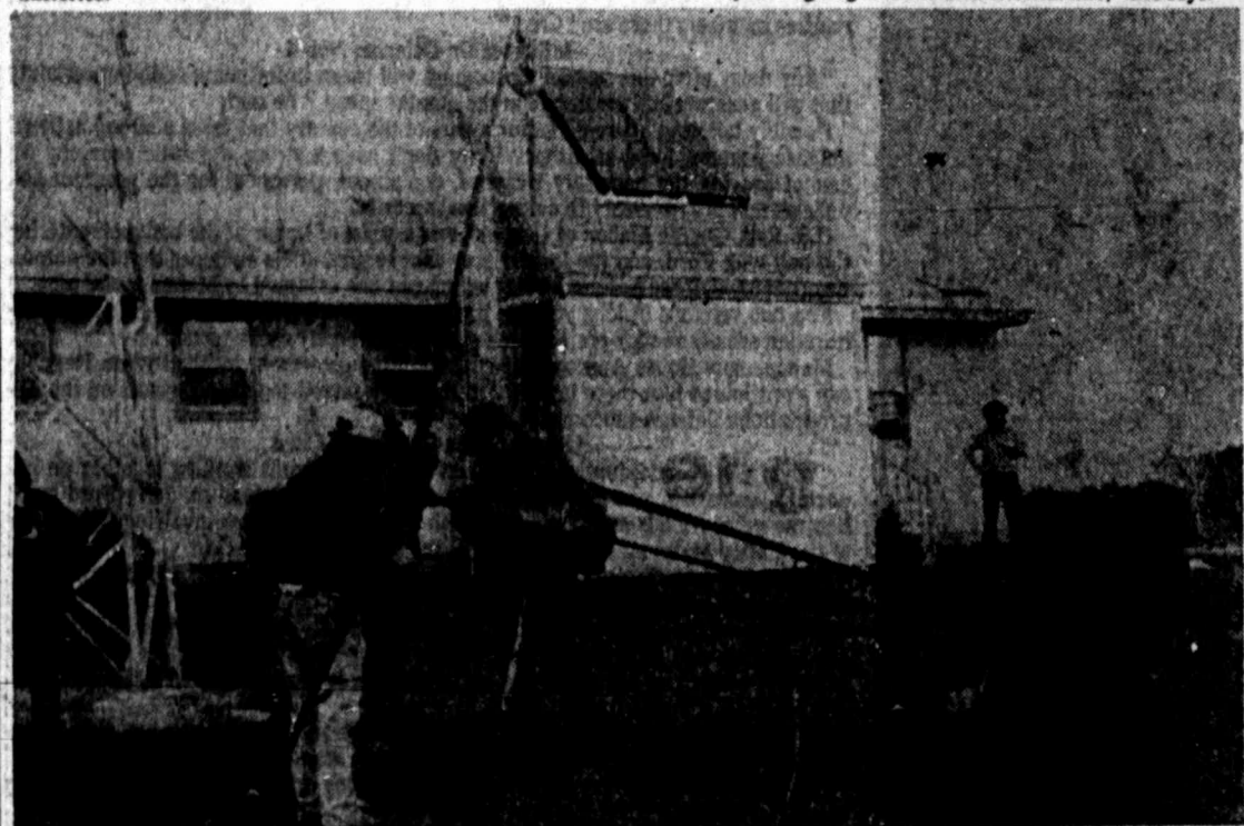
AERO WHAT?—Workers put the finishing touches on a wind generator in Williston Vt. The generator, which was hoisted atop a 40-foot tower, resembles a small plane and features propeller blades twice as long as the height of the men making the adjustments. (AP Laserphoto)
