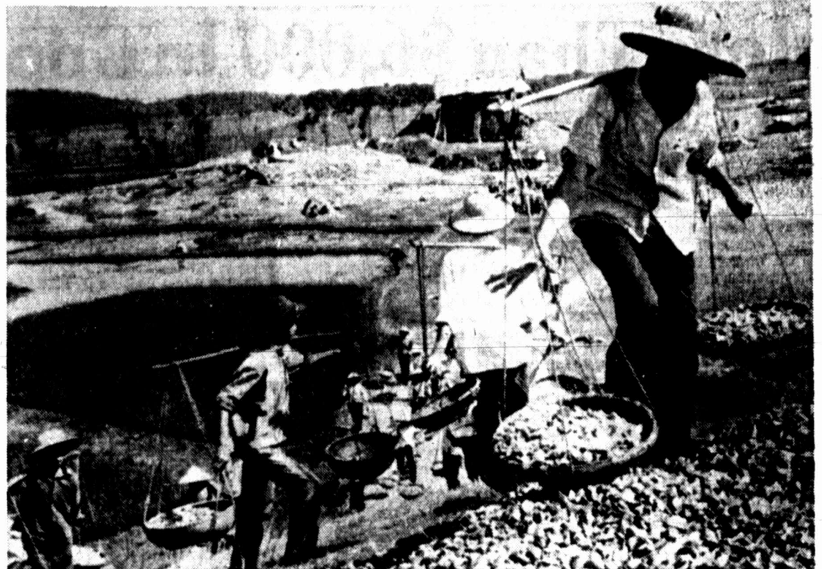
MANUAL LABOR — Vietnamese schoolchildren, 14-years-old and younger, carried gravel in baskets recently while working on a road along a dike near Thy Phuung. Due to a lack of earthmoving equipment and other mechanical aids, the youngsters had to perform the roadbuilding labor manually. The students spend one day each week on voluntary work supervised by their teacher. (AP Laserphoto)
