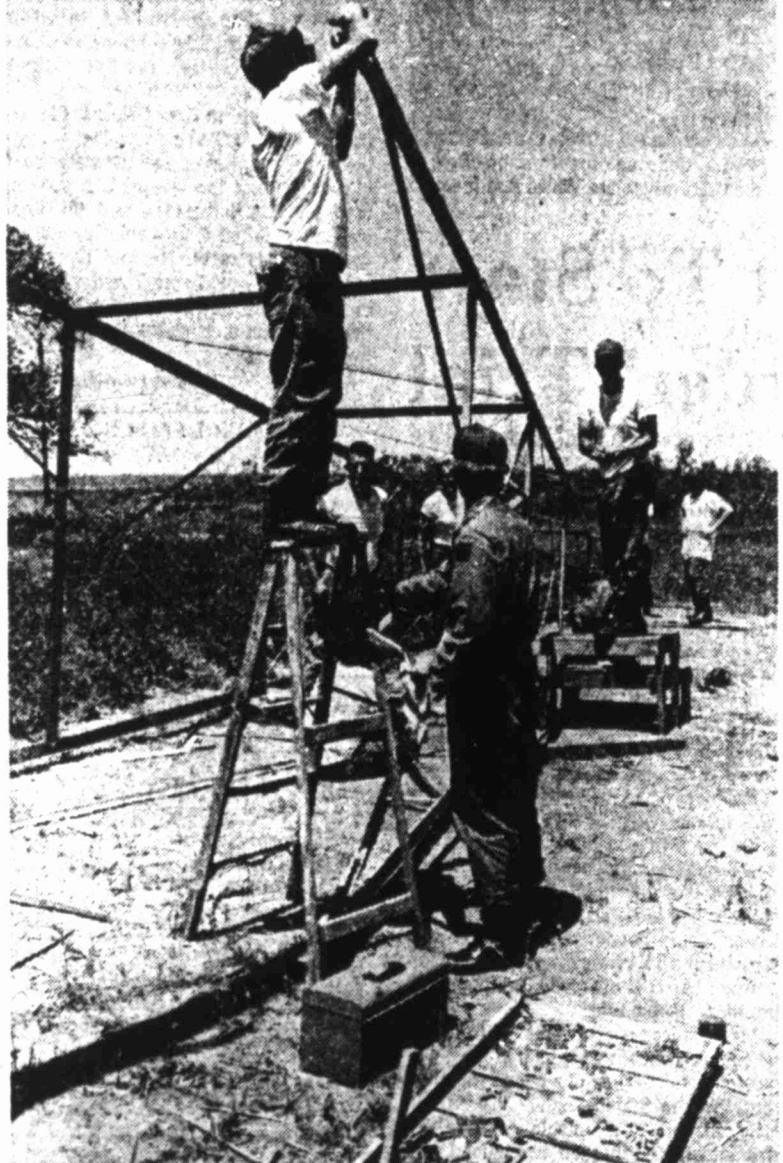
TILTING WINDMILLS — Army reservists from the 413th Civil Affairs Company assemble a windmill tower for Treehouse Village, a foster home for girls to be located west of the Lubbock Lake Site. The 40-foot tower, supporting a mill 14 feet in diameter, will pump water from 150 feet underground for the home, which will also be solar heated and cooled by wind-generated electricity. The dozen men have worked on the windmill tower twice in the past two months and hope to have the tower erected by the end of October. The company welcomes other similar projects, as long as the beneficiary is a non-profit organization. (Army Photo by Sgt. Dan English)
