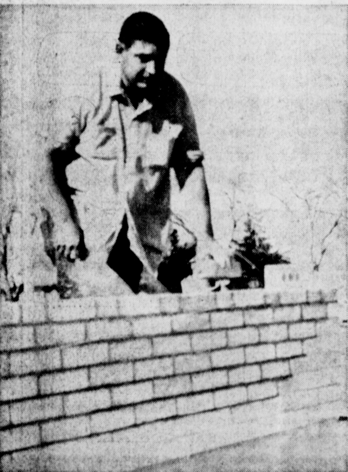
BRICK FOR DESHAZO - Construction of walls for the new DeShazo Elementary school structure has reached the brick-laying stage. This is one of the brick-layers at work, Charles Cobb, Amarillo.
