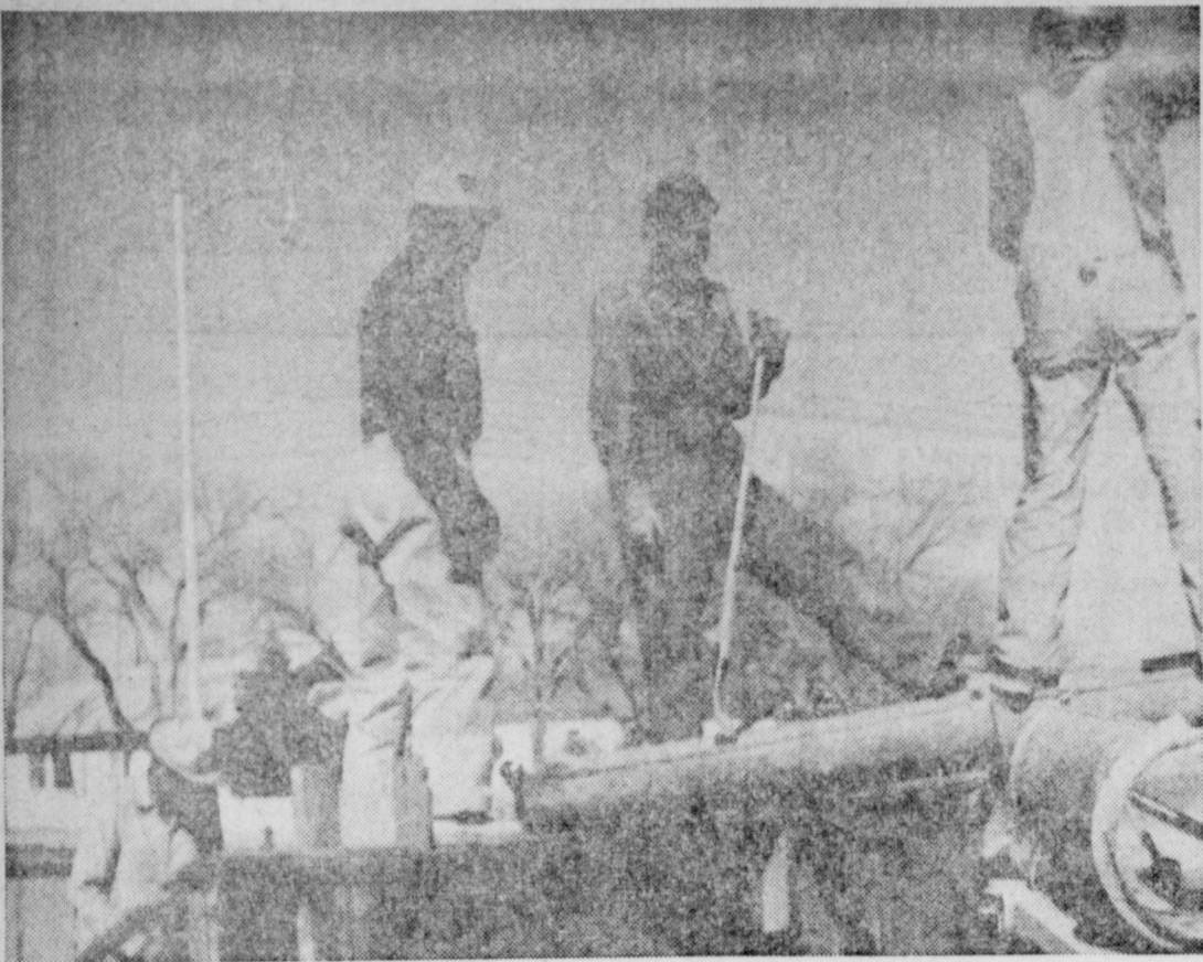
FOUNDATION GOING IN - L. to R. Ellis Sterling, Harold Brown, Hugh Rush, and Ocell Diggs are busy at work pouring the foundations for a new classroom at Mary DeShazo elementary school.
