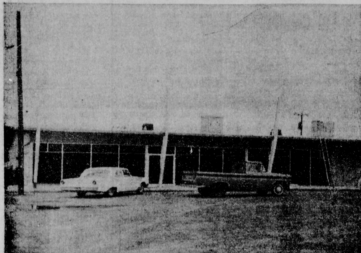
NEARING COMPLETION: The new home of Johnson Furniture Company is beginning to take shape as the building nears completion. Grand Opening for the new building is now set for October 11. B. and C. Construction Co. of Muleshoe, began construction July 26.
