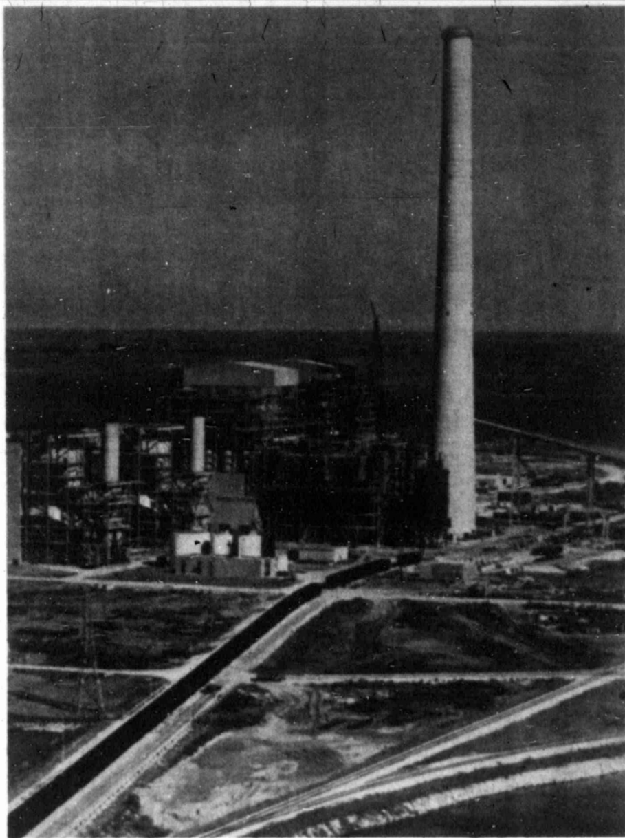
THIS GLEAMING CONCRETE smokestack, towering 700 feet above the rolling countryside, symbolizes San Antonio's determination to curb its addiction to increasingly scarce and expensive gas. The stack is taller than Tower of the Americas, is visible for 20 miles, and is being built at a cost of $326 million. It is part of a coal power plant. (AP Laserphoto)
