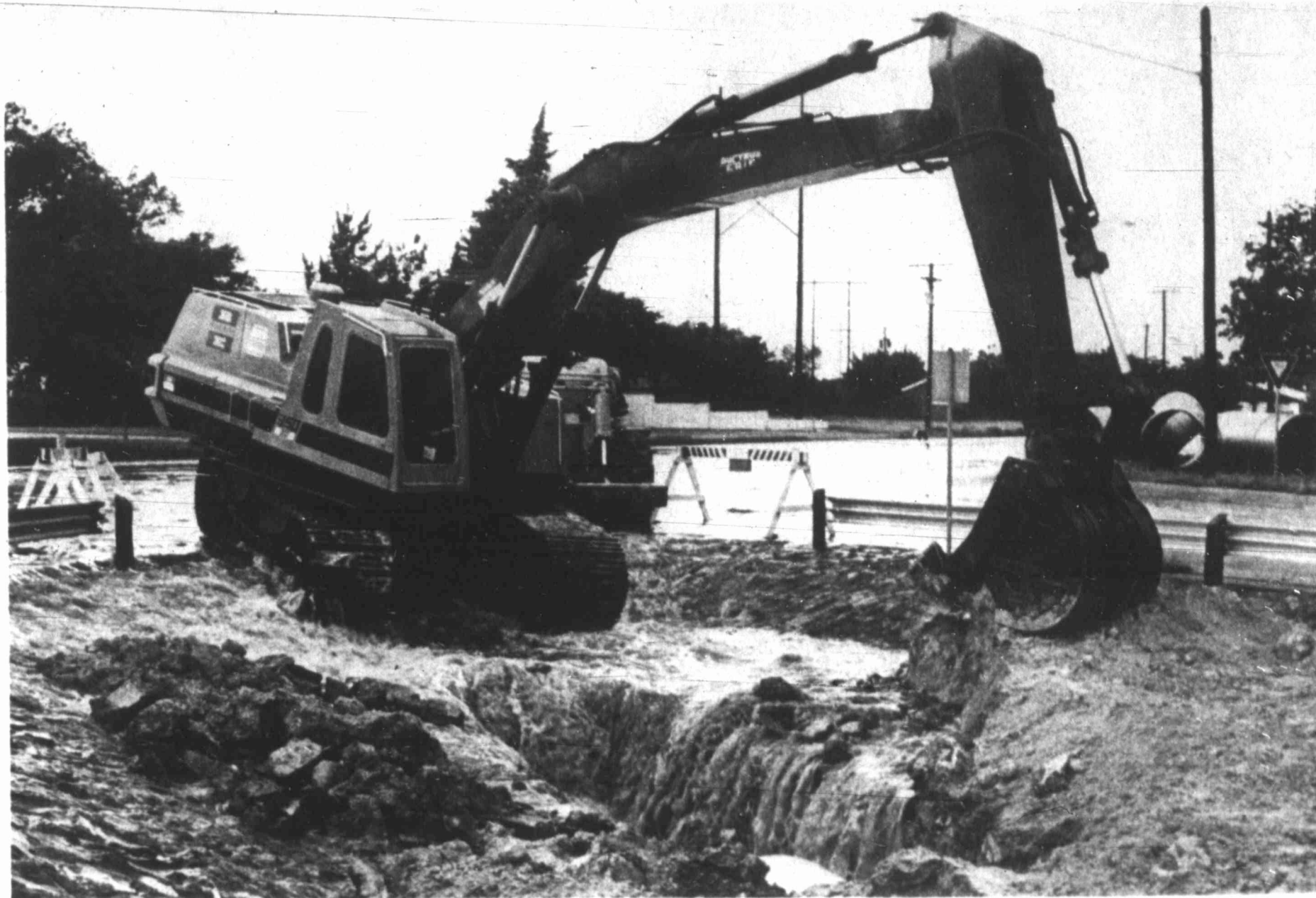
A dirt shovel at Scharbauer Drive and Golf Course Road looks like it may be washed away during Tuesday's rain.
