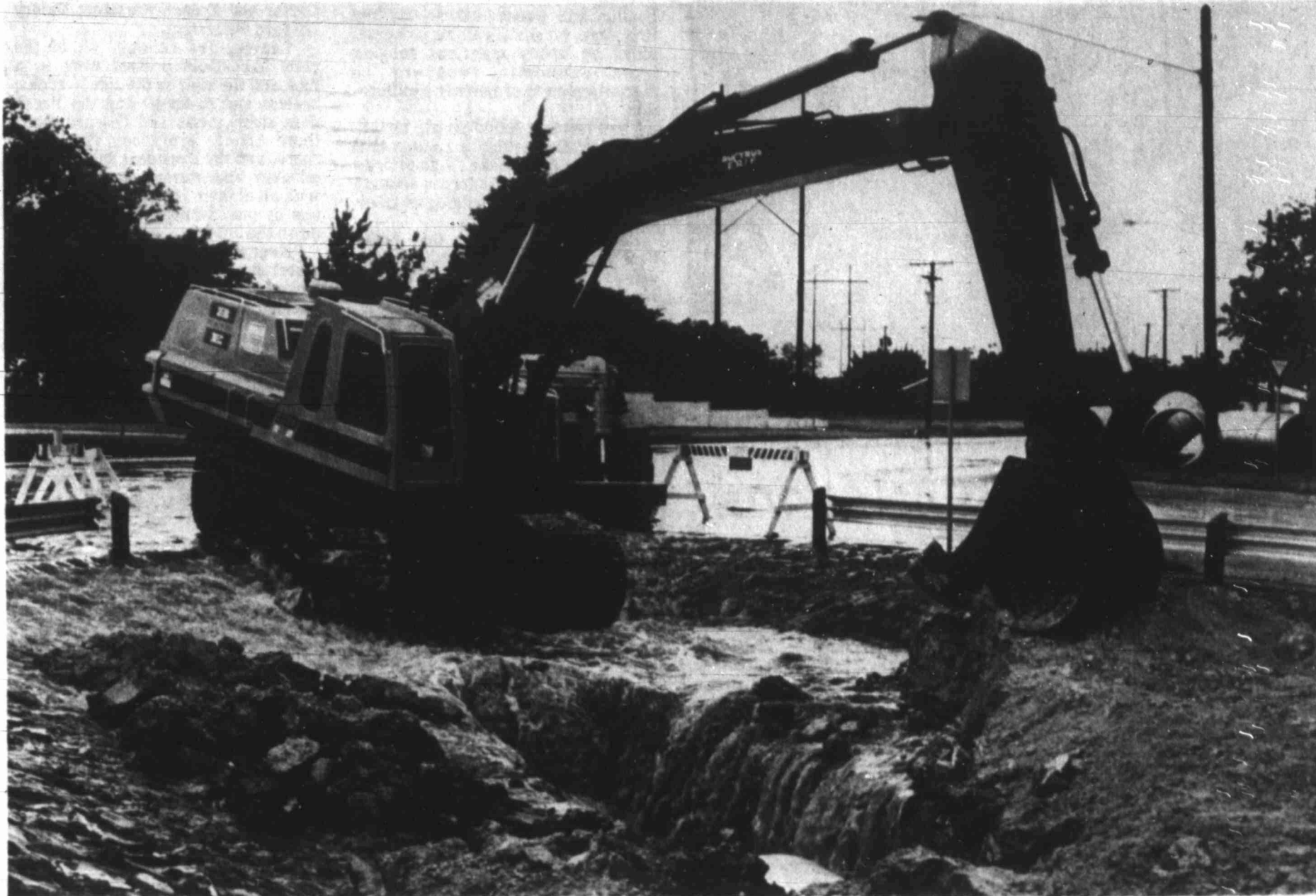
A dirt shovel at Scharbauer Drive and Golf Course Road looks like it may be washed away during Tuesday's rain.
