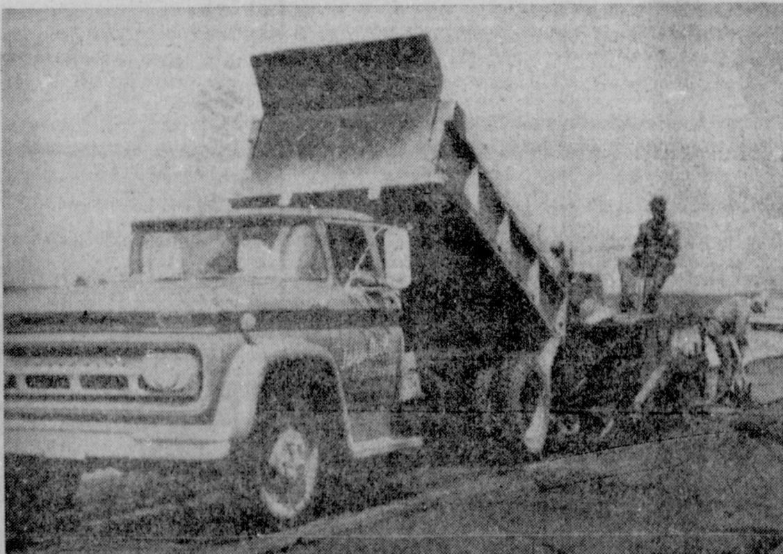
FINISHING TOUCHES — This machine is putting the finishing touches to the runways at Muleshoe airport. The second coat of Uvalde Rock is being applied and rolled with the machine behind the truck as it slowly makes it's way toward the end of the strip on the final run. A packing machine followed this one on the ground. (Journal Photo & Engraving)
