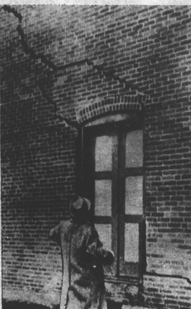
More than 4,000 persons left their homes in Shenandoah, Pa., when a 24-block area of the city sank into mine diggings. Damage is estimated in excess of $1,000,000. Shown above is a resident watching the ever-growing crack in the side of the depot as the ground level slowly changes.
