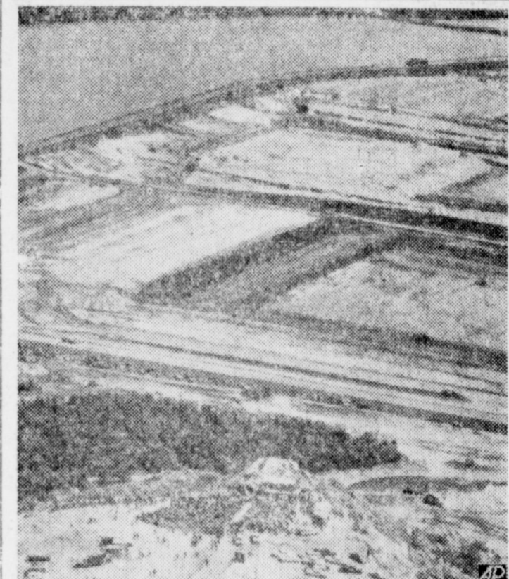
WEST TEXAS DAM — This is an airview of the Canadian dam site near Stanford in progress. Foreground shows ground-breaking ceremonies on a bluff overlooking the dam that will back water 28 miles in the Texas Panhandle. Background shows a coffer dam which rings construction in the river bed. (AP Photo)
