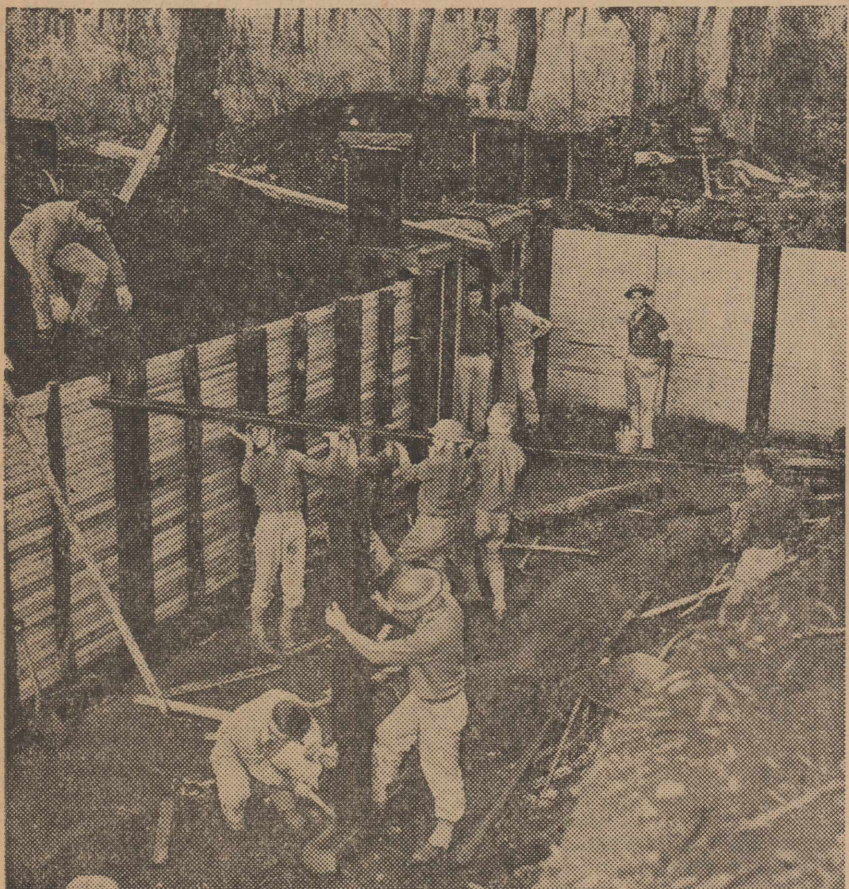
U. S. troops and native workmen work on underground installations of dugouts. This is a first aid dugout equipped to perform surgery in an advanced position.
