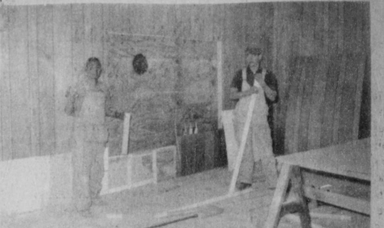
REMODELING: After just a few days of work, Martin's Grocery Store is already beginning to take on a new look. Shown in photo at left is Tony Yanez and Buster Wright putting up new panneling. Martin Soliz, owner of the store, said that work was expected to take about 2 weeks.
