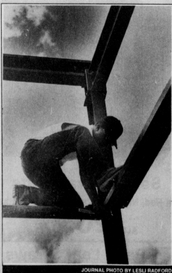
Contractor Joe Medellin bolts a beam in place Thursday as construction of the new Muleshoe High School band hall moves along.
