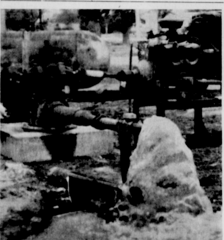
The new City well, drilled to 650 feet, was pumped in this week at 125 gallons per minute. A 350-gallon well had been hoped for, but the new well will help with the local water situation at present. The City will ask for bids on a pump for the new well in the near future.
