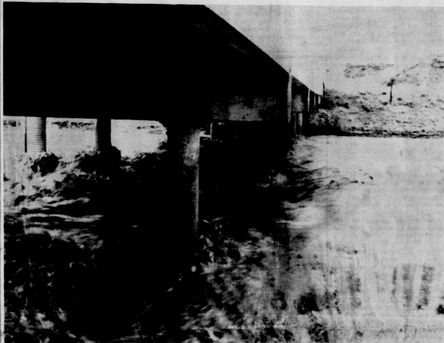
Tule Creek floodwater crested at 11.5 feet at about 8:30 a.m. Friday. Many acre feet of water have gone down the creek toward Lake Texoma since the first of June. —Briscoe County News Photo
