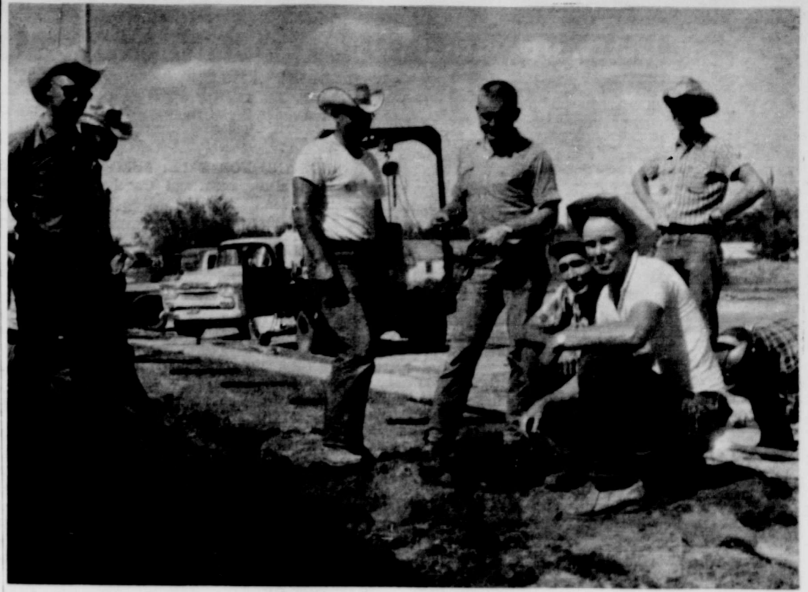
The Silverton Young Farmers chapter has recently completed the installation of a railing around the sidewalk at the new school cafeteria for the protection of the grass which has been planted. Pictured taking part in the project are Joe Brannon, Ronald Dale Kitchens, Robert Haley Hill, Wayne Stephens, Jaye Turner, G. W. Chappell and Gordon Lowrey. Also assisting with the project were
