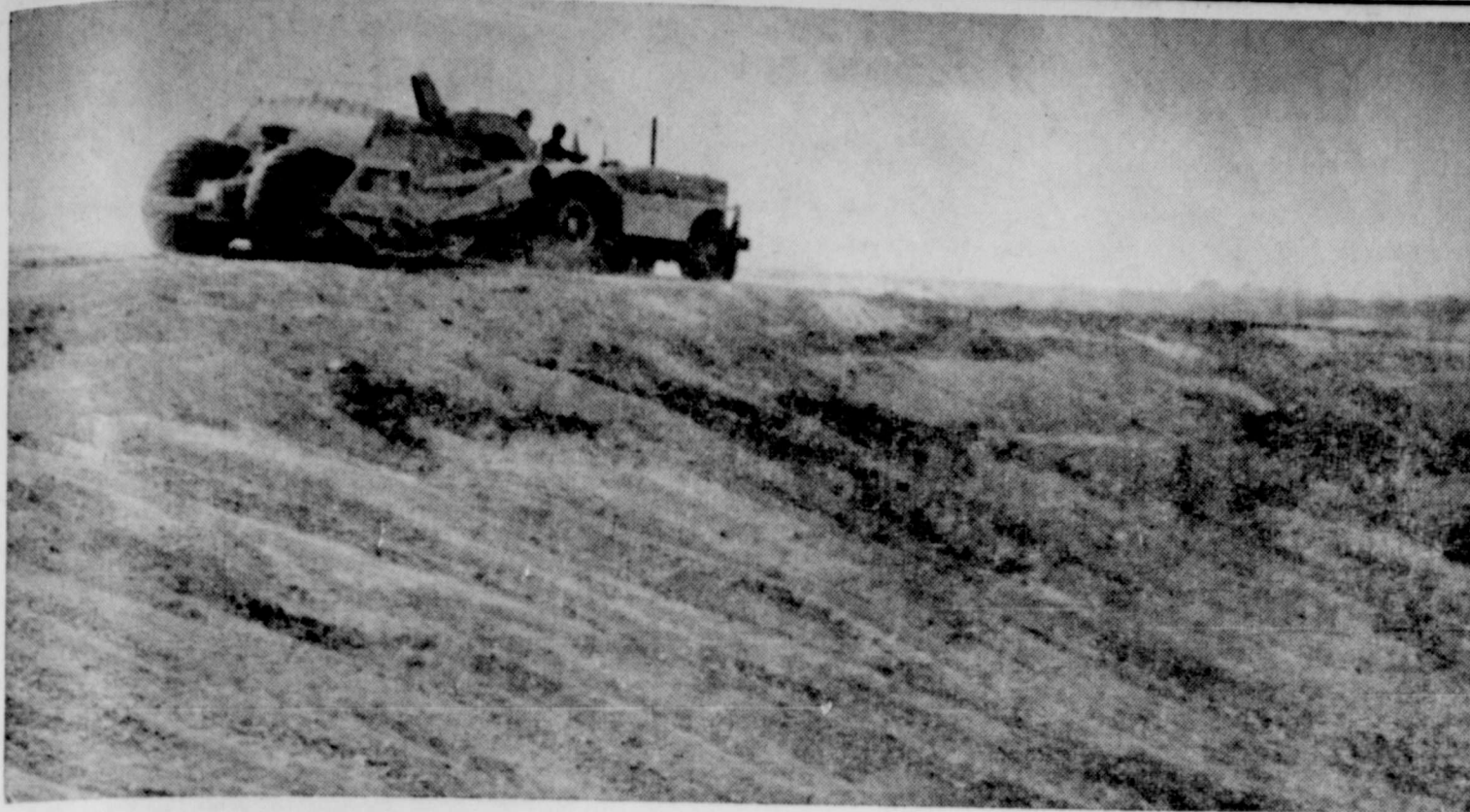
The above picture shows construction of an erosion control dam on the Tom Barbee farm Northeast of Quitaque. This dam is only one of the many practices scheduled by Barbee under his Great Plains Program plan. The main purpose of this dam is to protect a field below which will now be terraced. It will store about thirty-two acre feet of water. The spillway will function only about once in fifty years, which
