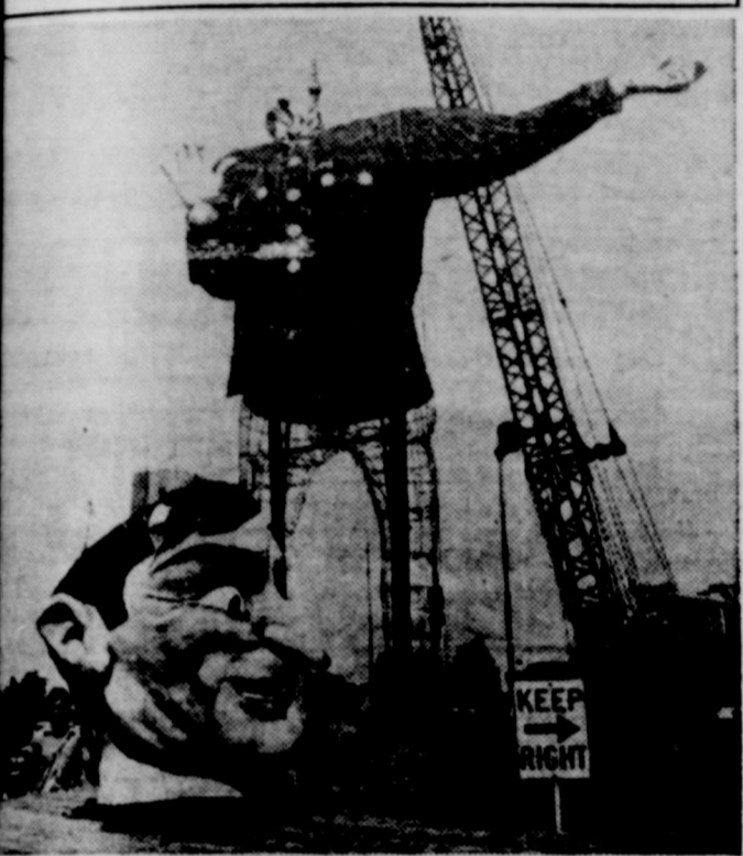
"Big Tex," the towering 52-foot cowboy statue who symbolizes the great State Fair of Texas, is being put together in readiness to welcome some two-and-a-half million visitors to the 1958 exposition, October 4 through 19, in Dallas. It takes a crew of workmen with a 100-foot derrick to put the big boy's head on his shoulders.
