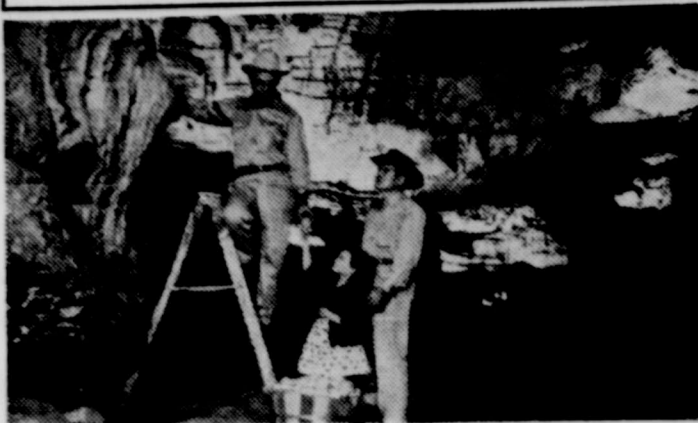
A completely new and improved lighting system has just been installed in Texas Longhorn Cavern near Burnet which provides dramatic illumination designed to best show off the scenic wonders of this marvel of Nature. Many modern theatrical lighting effects have been utilized. More than four miles of wiring were installed and nearly a thousand electric bulbs were used in the project which required over five months.
