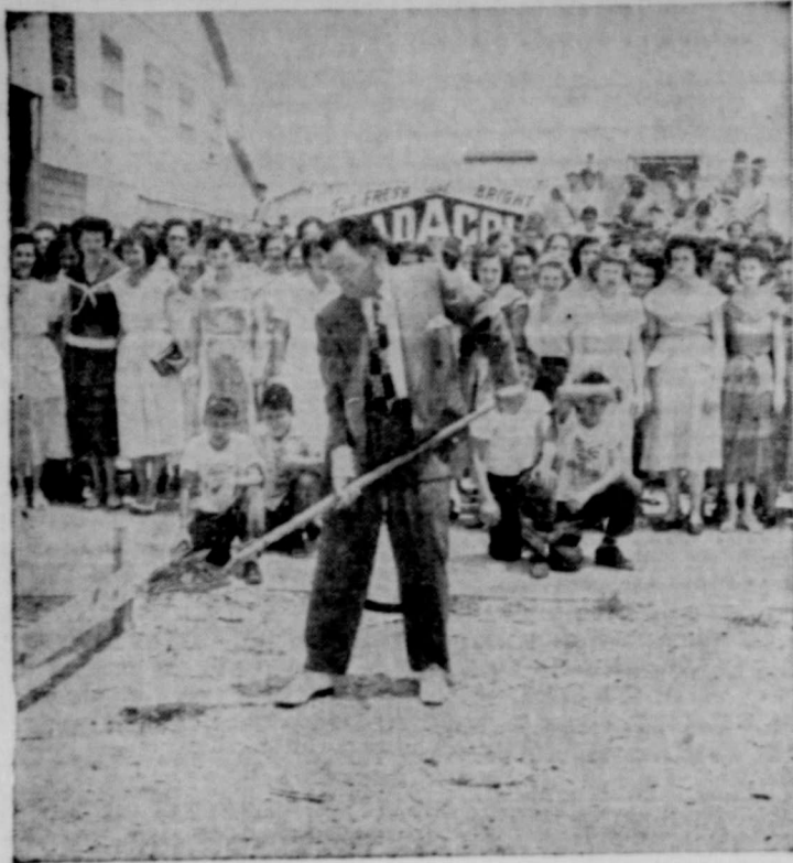
Senator Dudley J. LeBlanc, creator of famous HADACOL is shown above breaking ground for the new HADACOL factory now being built alongside the present plant in Lafayette, Louisiana. This new building will be 80x225 feet, two stories, steel and concrete construction. The remarkable growth of HADACOL has forced the immediate construction of this new building. Only last spring Senator LeBlanc opened the present HADACOL plant and now less than a year later, HADACOL requires a 100% increase in factory space.
