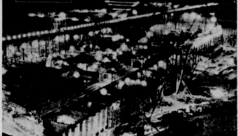
WORK goes on day and night at Grand Coulee dam on the Columbia river in eastern Washington, where the U. S. is building the world's most massive masonry structure.
