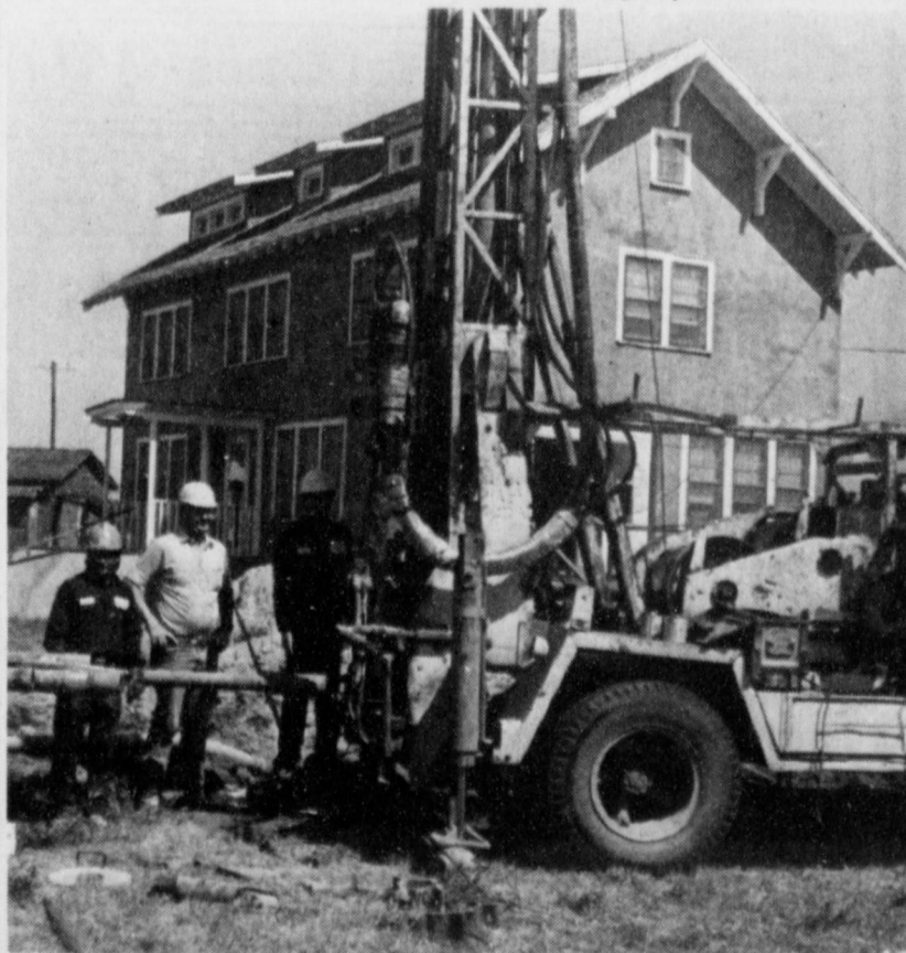
HERITAGE COMPLEX GETS WATER WELL ---Stanley and Patricia Wilson donated the drilling of a water well to the Heritage Complex. The well was dug Monday morning. Pictured are workers of Wilson Drilling. (Journal Photo)
