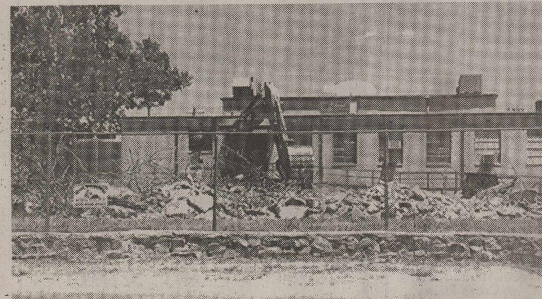
Tearing Away the Old - The old tennis courts near the cafeteria were removed to make way for the new Elementary Gym and Tornado Shelter.
