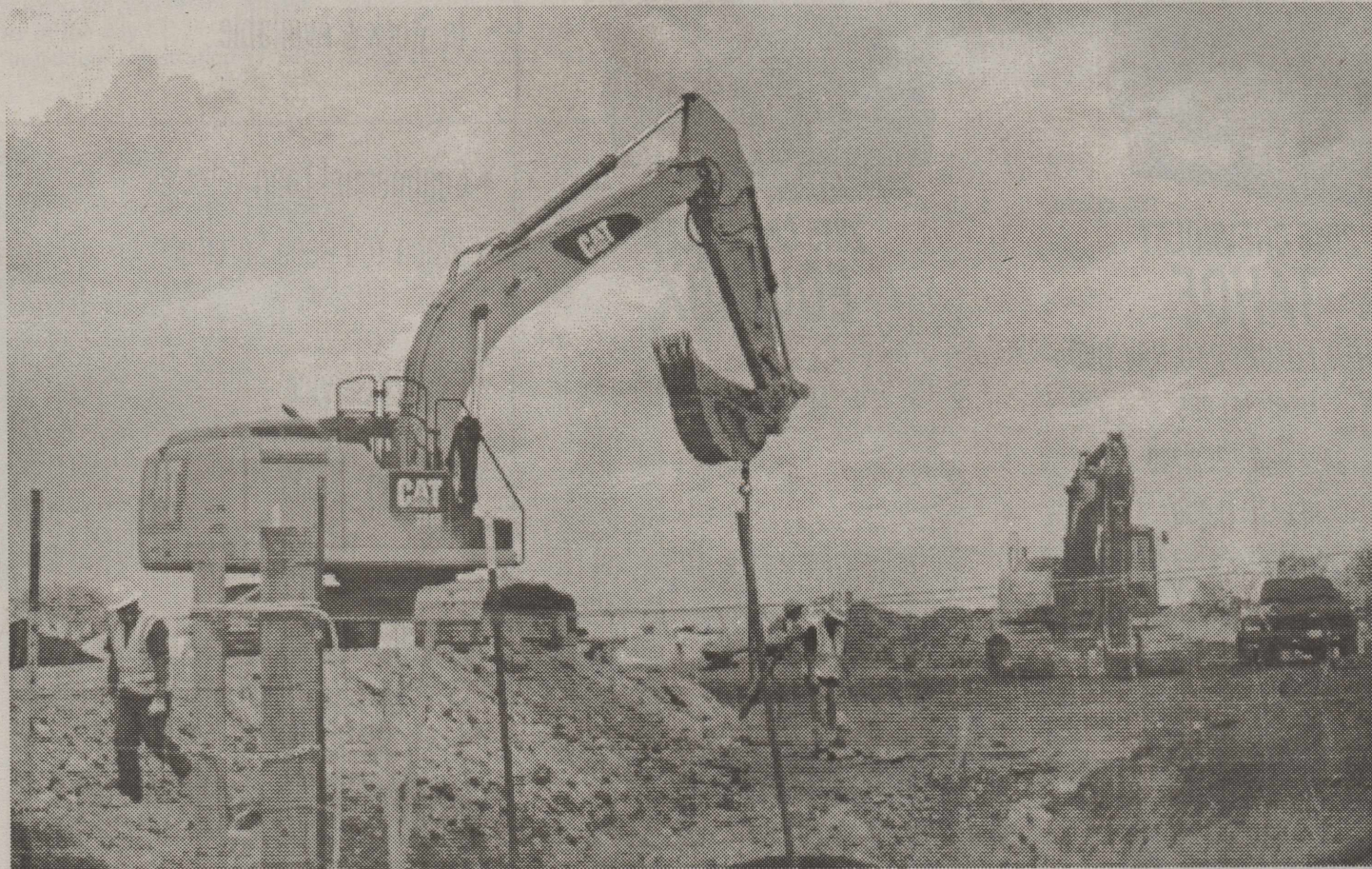
PIPELINE CONSTRUCTION — A pipeline construction crew was working on placing two 12 inch pipelines under FM 603, just north of the Eula community in Callahan County on Wednesday, September 9th. Two 12 inch oilfield-related pipelines are now
