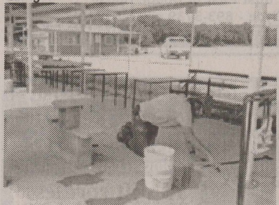
CALLAHAN CO. 4-H—Bill Cedergren working on the concrete pour at the range.
