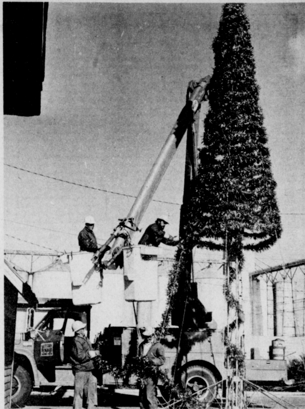
PUTTING UP THE TREE--Each year, workmen from Bailey County Electric Cooperative put up the Christmas tree at the Mule Memorial. This year was no different. Here, Seth Shaw and Mike Roberts in the buckets and Vernal King and Bill Wilkins on the ground are busy putting up the tree which will be lighted nightly during the holiday season. Street decorations were also put up Thursday, to help brighten the town for residents, and for travelers.
