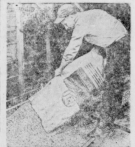
Zonolite vermiculite insulation being installed over ceiling of dairy barn at Mississippi Farms, Oregon, Ill.
