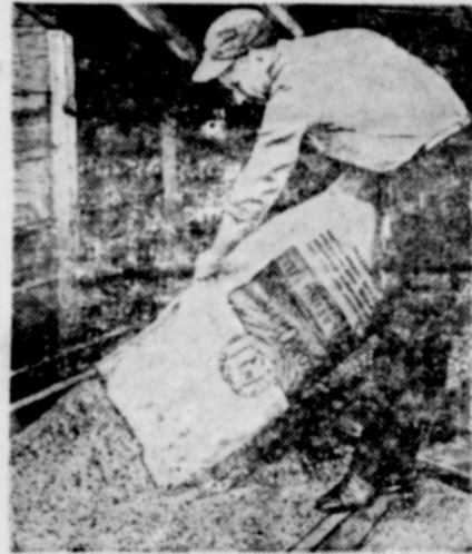
Zonolite vermiculite insulation being installed over ceiling of dairy barn at Sinnissippi Farms, Oregon, Ill.
